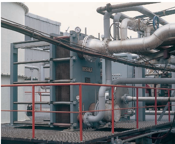
Solvent recovery, exhaust gas cooling
