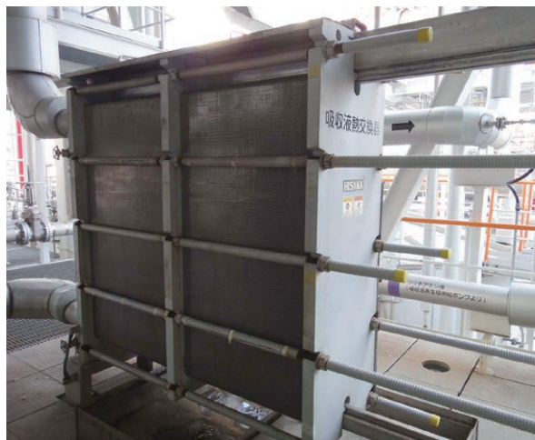
CO 2 recovery, desulfurization plant solution heat exchange
