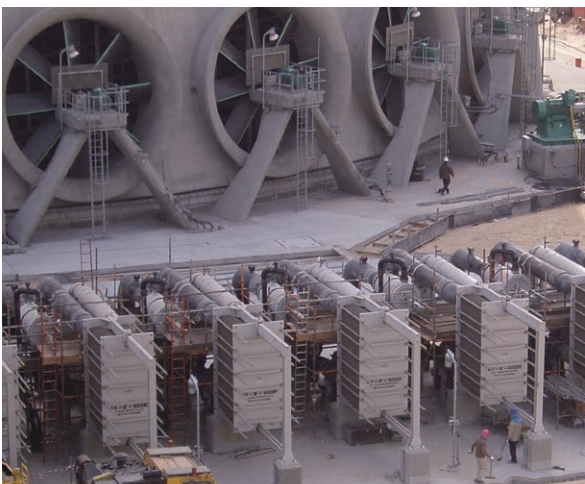
Central cooling system
