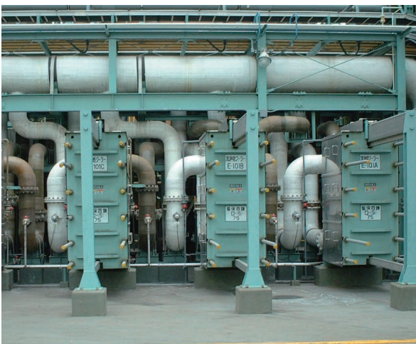
Sulfuric acid, electrolytic plating cooling
