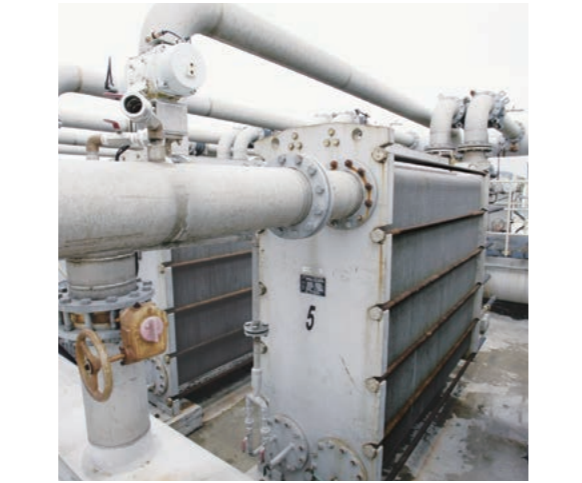
Heat exchange of black liquor / white water, oven blow gas condensation, waste heat recovery
