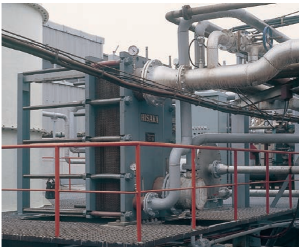
Solvent recovery, exhaust gas cooling
