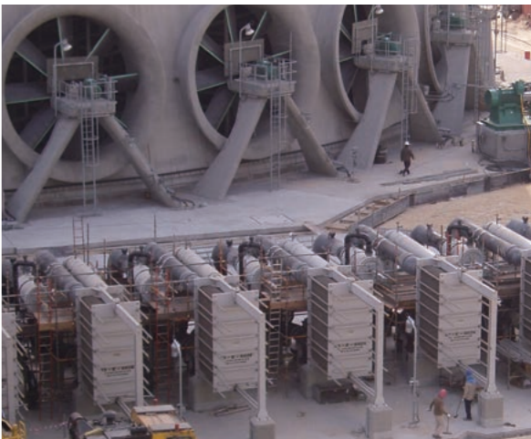
Central cooling system
