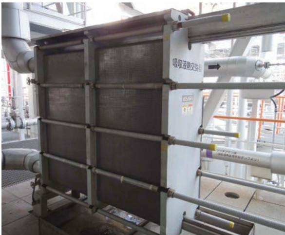
CO 2 recovery, desulfurization plant solution heat exchange
