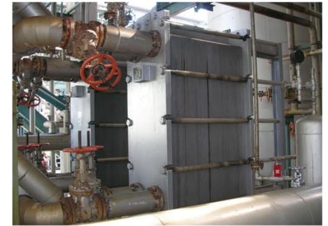
Rich/Lean Amine Heat Exchanger
