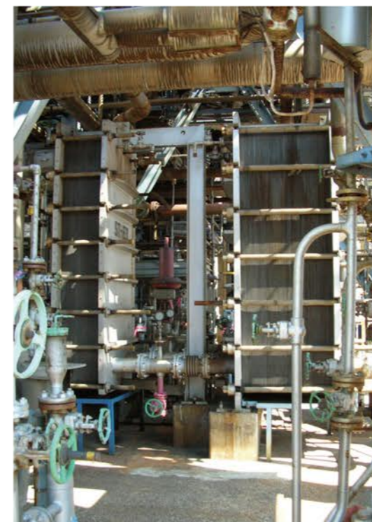
MDEA Heat Exchanger
