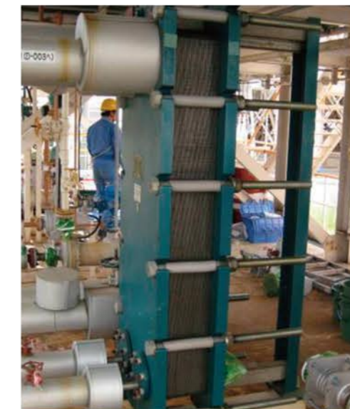
Rich/Lean Amine Heat Exchanger
