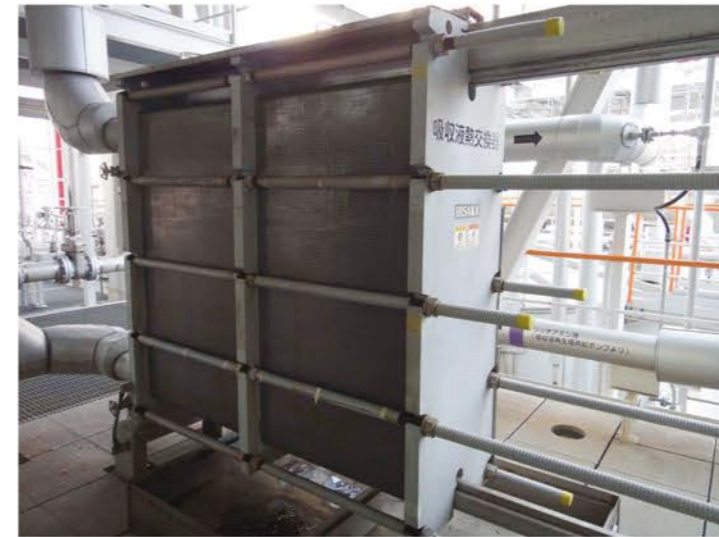
Rich/Lean Amine Heat Exchanger
